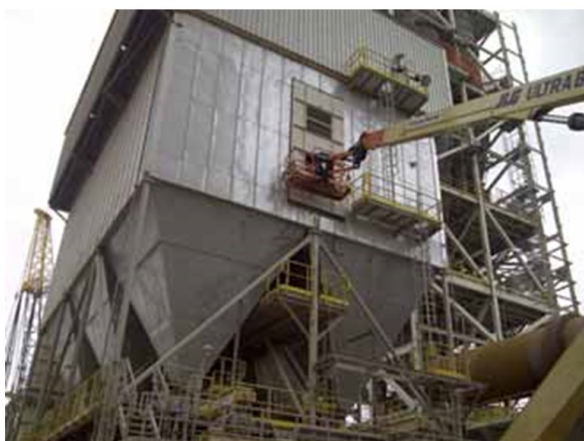
Kiln/raw mill filter: internal deflectors modifications.
