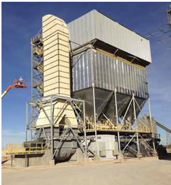
Kiln/raw mill filter: dustworks overview.
